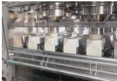
Positive pressure in the filling room maintains the hygiene conditions during filling operations in the food and pharmaceutical industry
